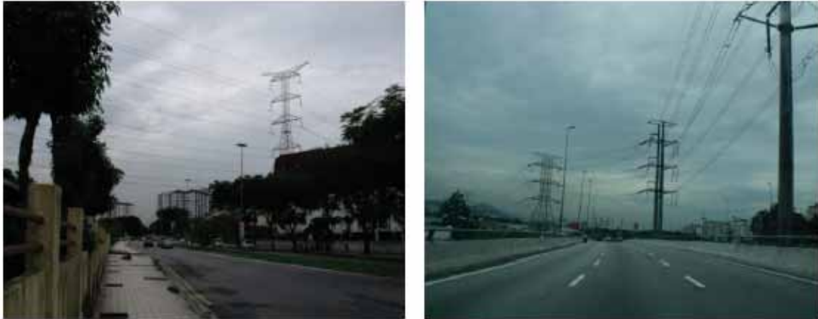
Figure 6: Picture of transmission lines above public road
